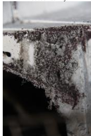
Fig. 4. Detail of a cage, an example of an insufficient efficacy of the liquid formulation based on SiO 2 in a housed facility.
